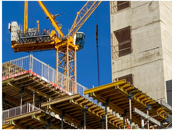
Tower crane alongside the construction of the lift shaft of a new office development in Cardiff city centre. © iStock
