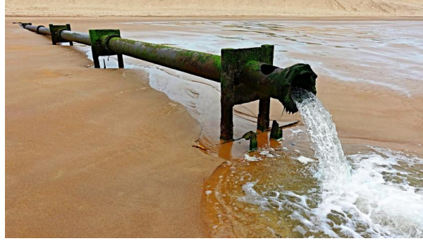
Water flowing out of sewage outfall pipe onto beach © Pixabay
