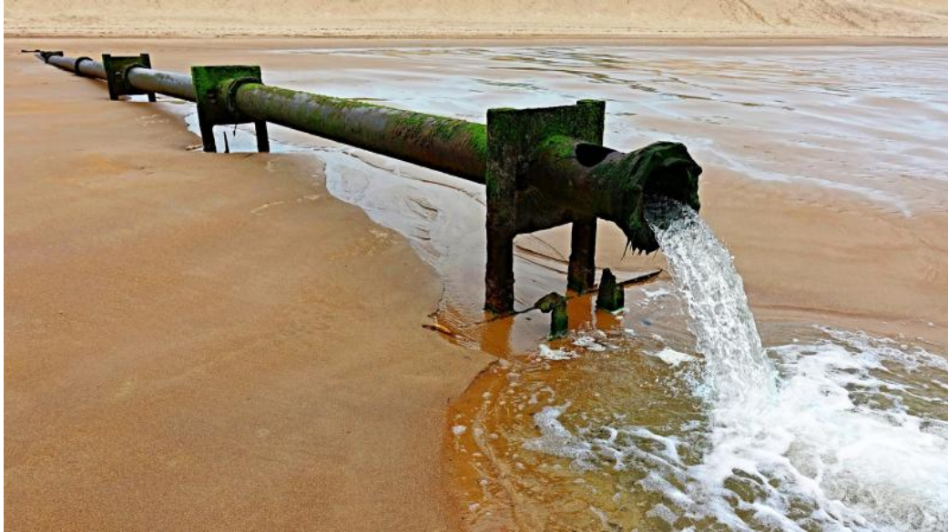
Water flowing out of sewage outfall pipe onto beach Pixabay
